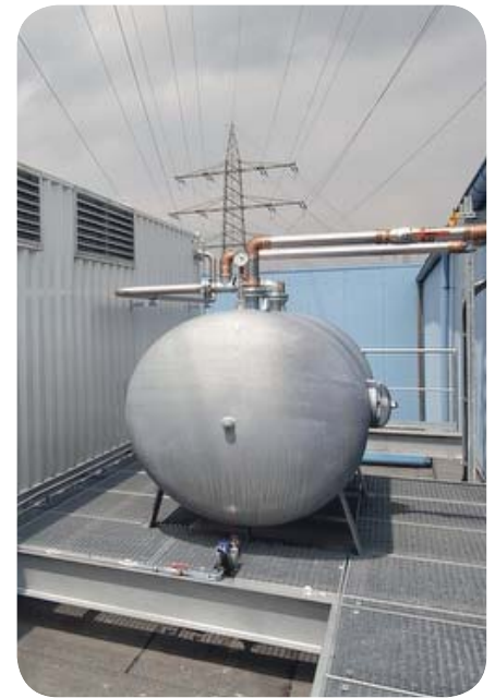
The storage tank was also installed on the roof.
