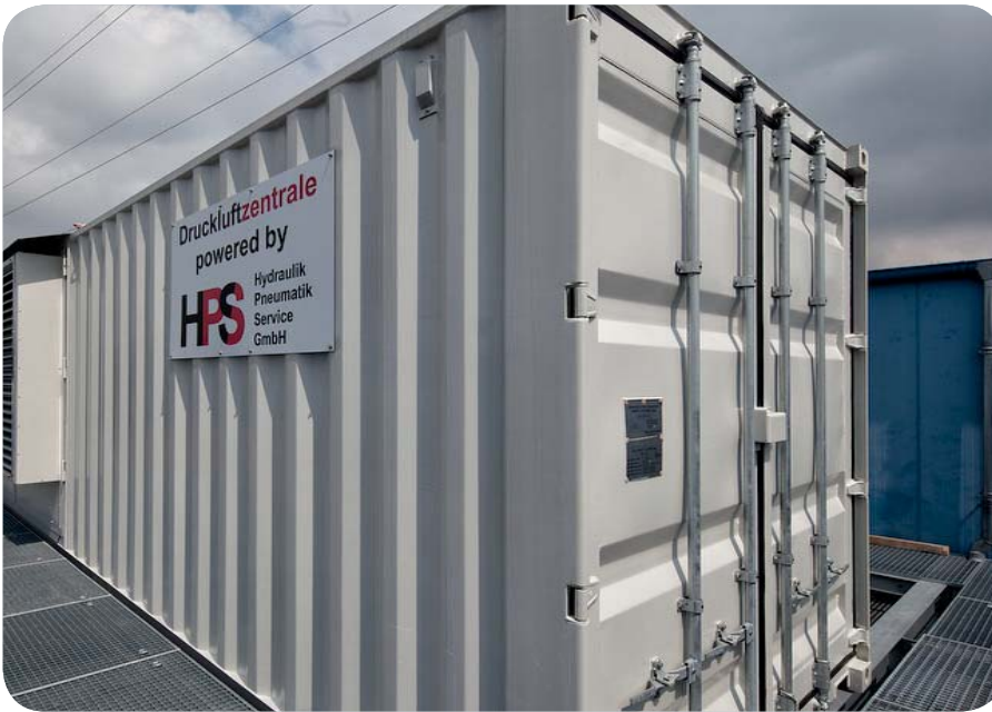
The container compressed air station is optimally located at a central point on the roof of a production building.
