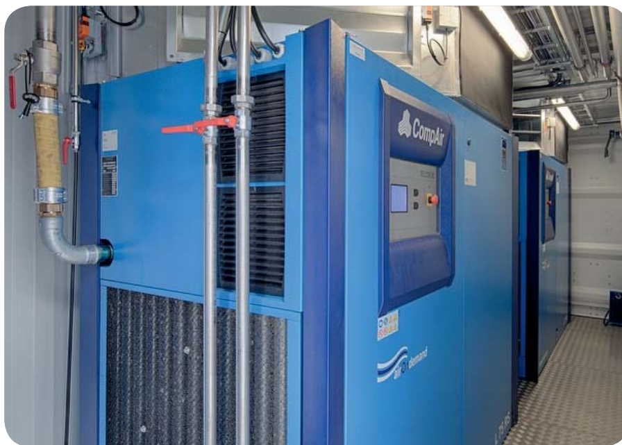
Three 75 kW regulated speed compressors generate the compressed air that the GDK factory needs.
