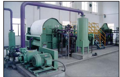
Drum Filter Vacuum System
