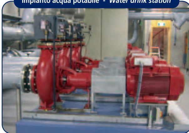
Impianto acqua potabile - Water drink station
