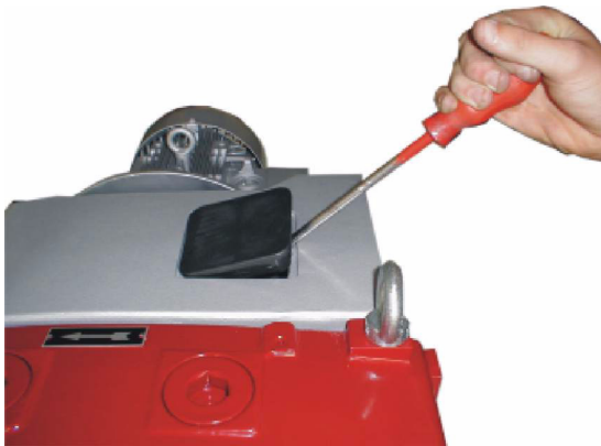
Figure 9.5 Cleaning the cooler
